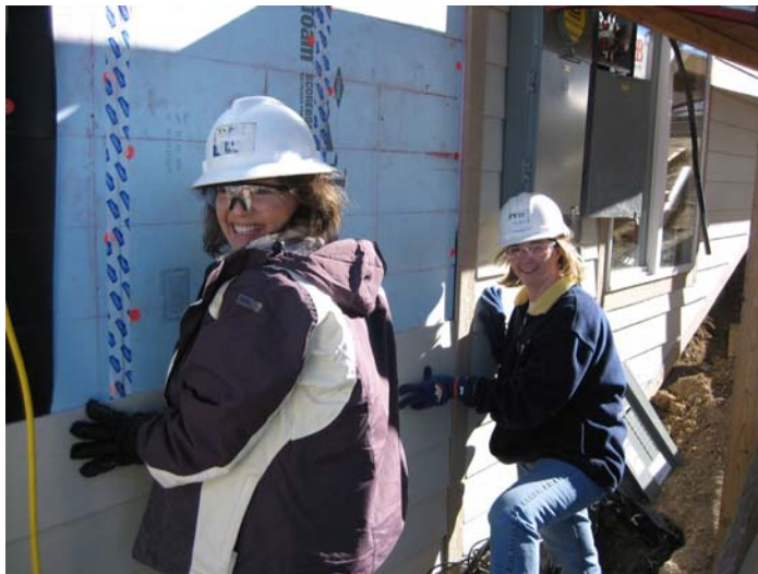
SunCorp employees Joanie Edquist (left) and Jill Robinson install siding while assisting Habitat for Humanity build duplexes.
